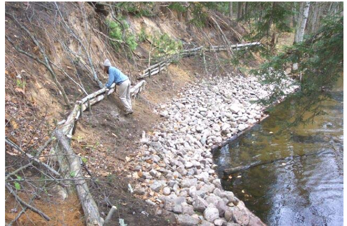
“ During – Fieldstone was placed at the toe of the bank, and the upper slope was terraced, brushed, and planted. “Edge logs” of the fish cover structures are just visible underneath the fieldstone.”
